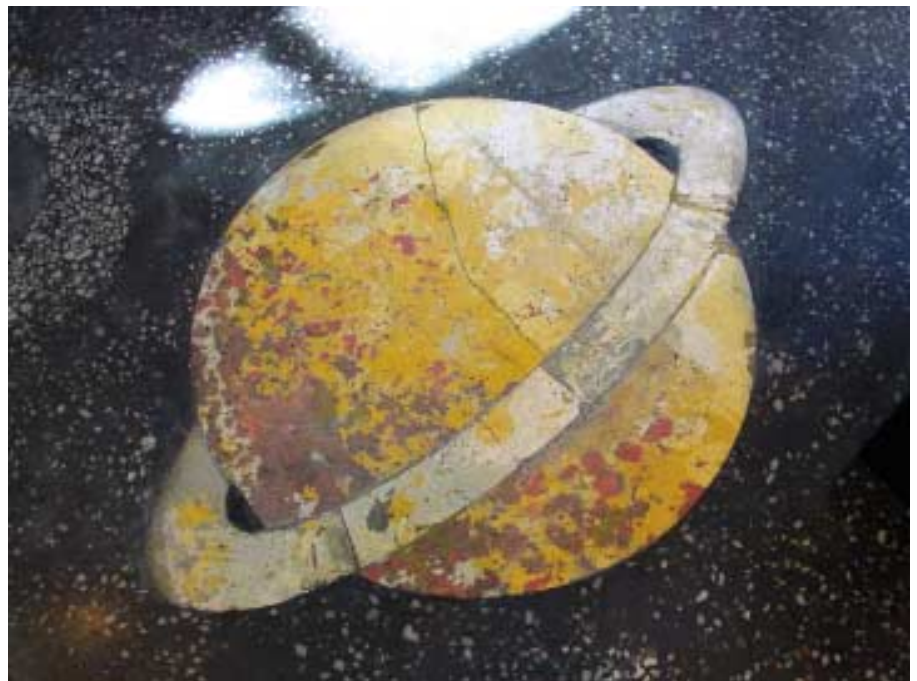
This ringed planet was precast with hand-packed integrally colored concrete “blobs,” then installed formed side up on a structural concrete substrate. The integral black field, with artfully scattered aggregate, was placed then ground. Cracks, patchy colors, and the sporadic nature of the aggregate exposure enhance this historic Italianate concept
